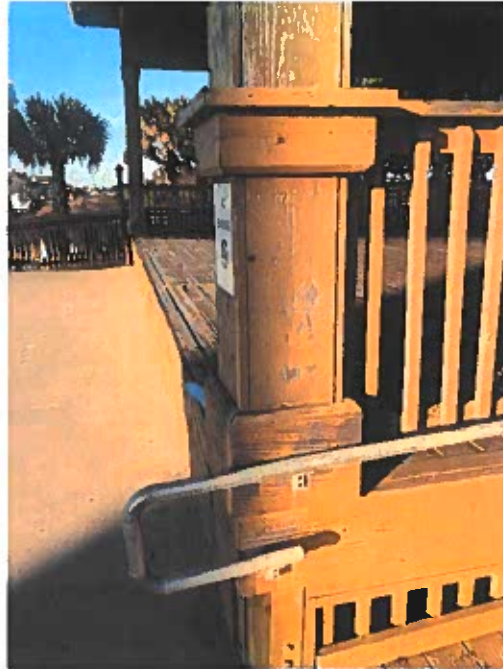
Photo 3 – Corner pile with no pile repairs
