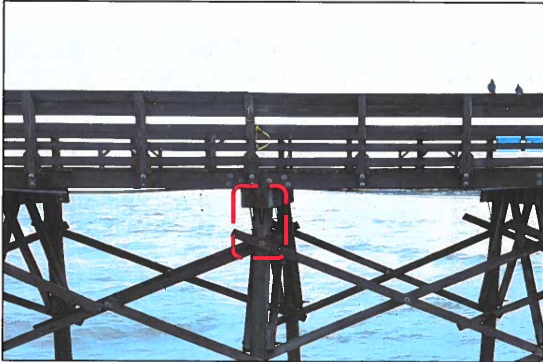
Photograph 5: Pile 40A - Top 18-inch pile is broke/overstressed
