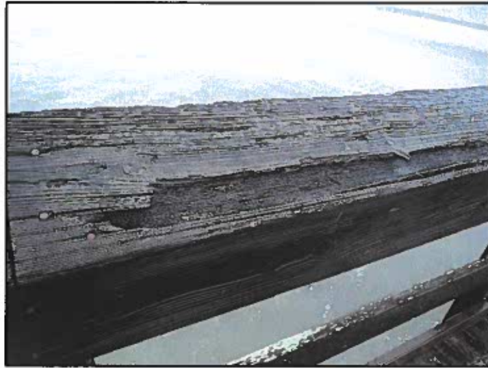
Figure 19. Example of railing in poor condition
