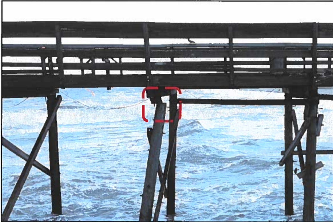
Photograph 3: Pile 24A - 50% Bearing due to displaced pile shims
