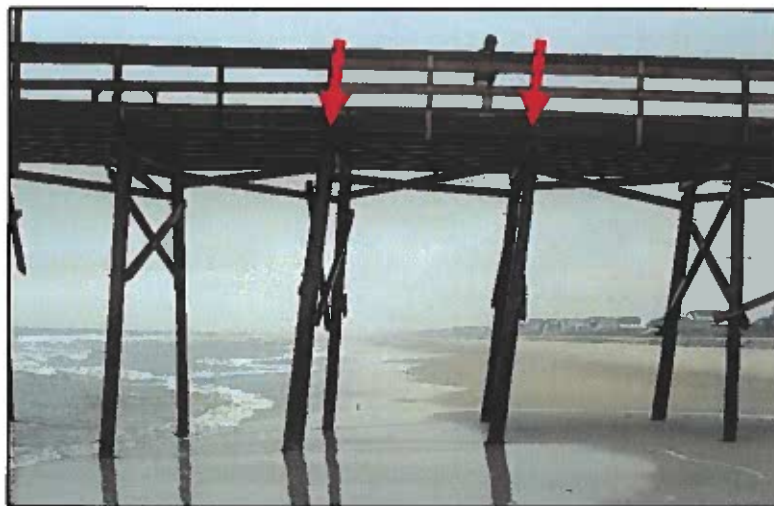
Figure 8. Photo of leaning piles nearshore
