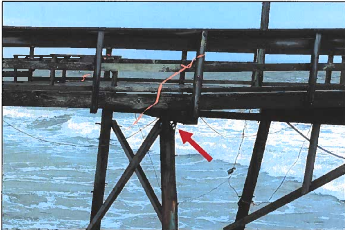
Photograph 4: Pile 25B - Top 18-inch pile is broke/overstressed
