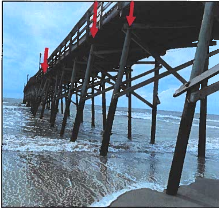
Figure 7. Photo of significant leaning of piles in two locations
