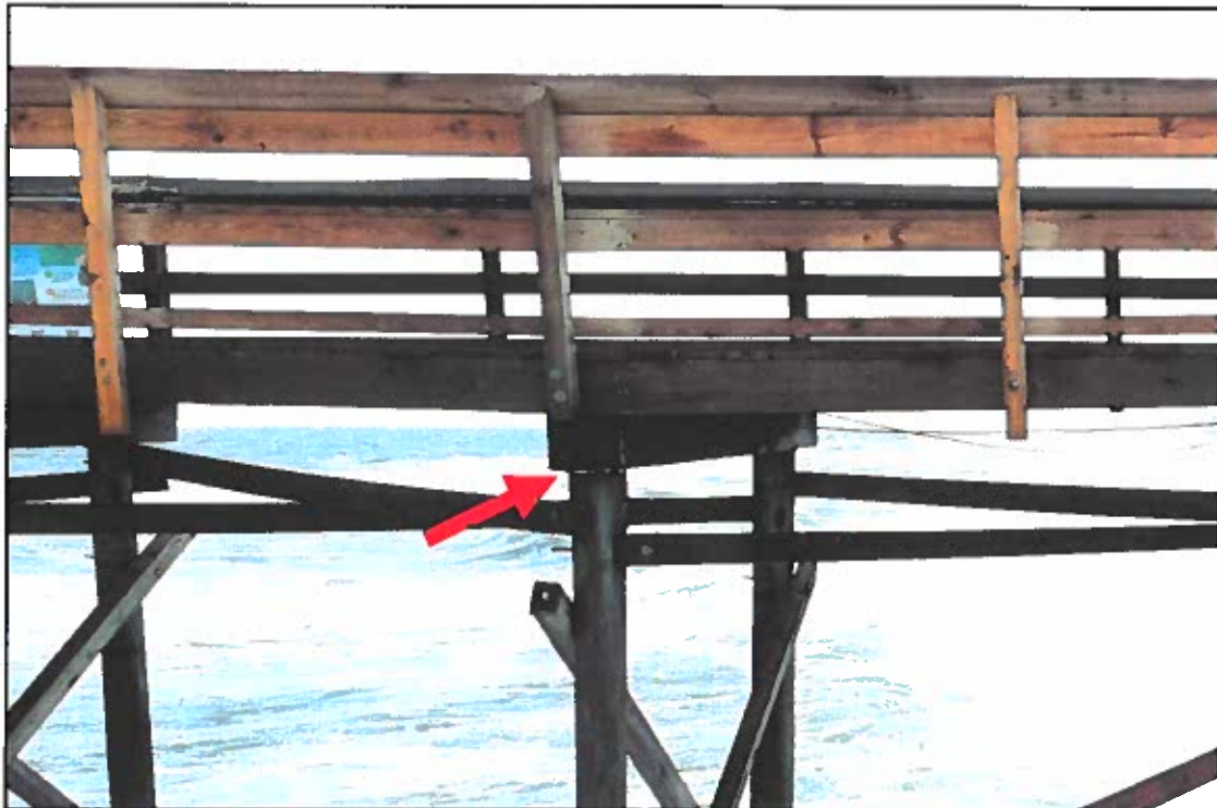
Photograph 2: Pile 17A - 100% Non-Bearing pile, timber cap supported by steel fish plates
