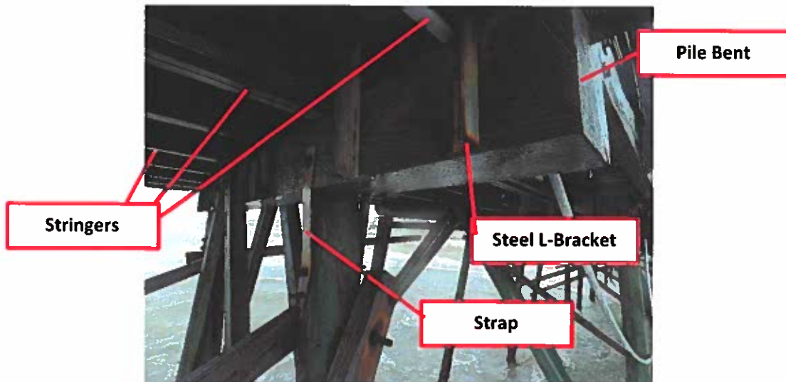
Figure 14. Example of stringers attached to pile bents by steel L-brackets with moderate corrosion (fair condition). Pile is attached to pile bents by straps.
