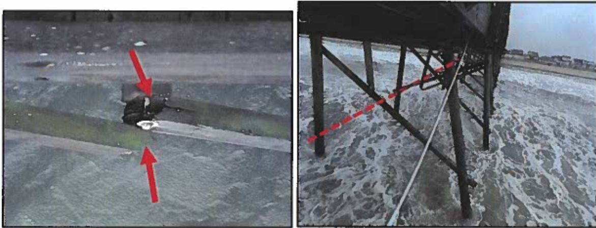
Figure 11. Example of broken cross-brace (left) and missing vertical cross-brace (right)
